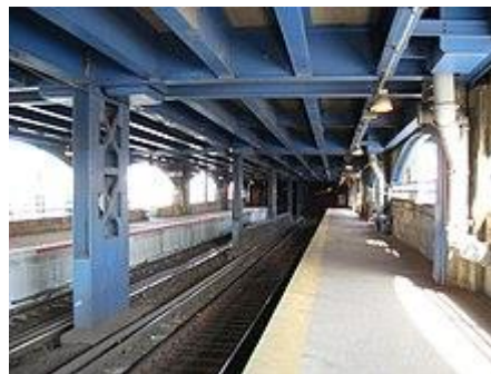
A view of the East New York station of the Long Island Railroad (LIRR), seen in 2008
