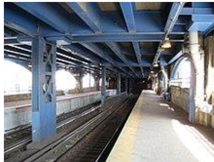
A view of the East New York station of the Long Island Railroad (LIRR), seen in 2008
